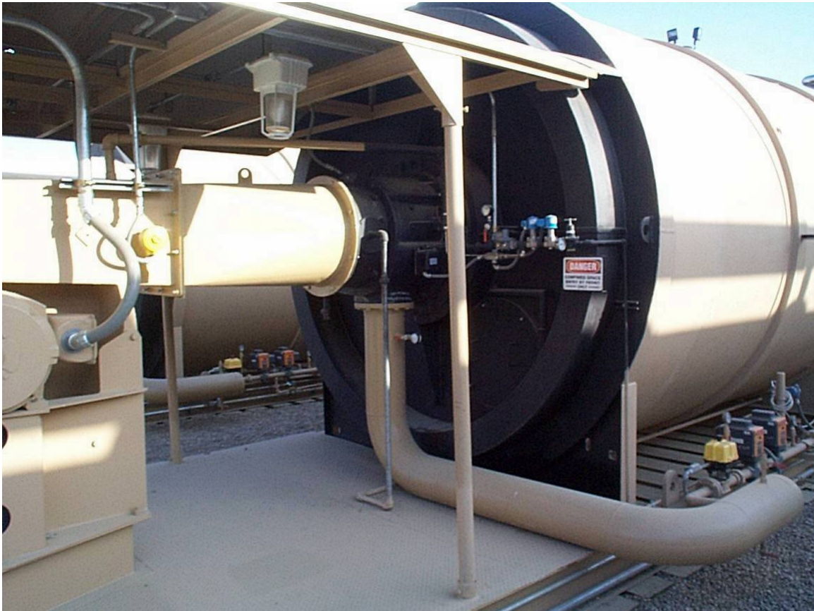
Blower and Burner Area
