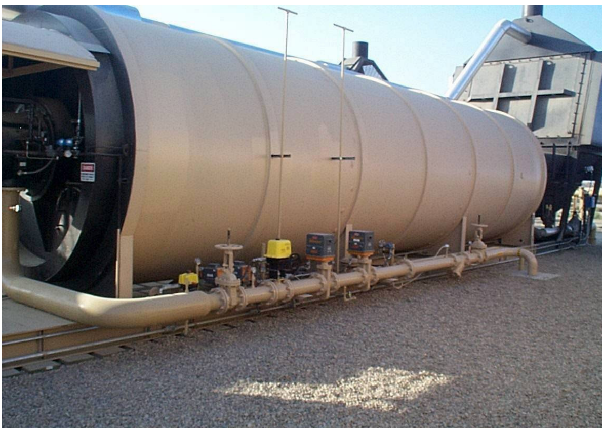
Fuel Gas Train
